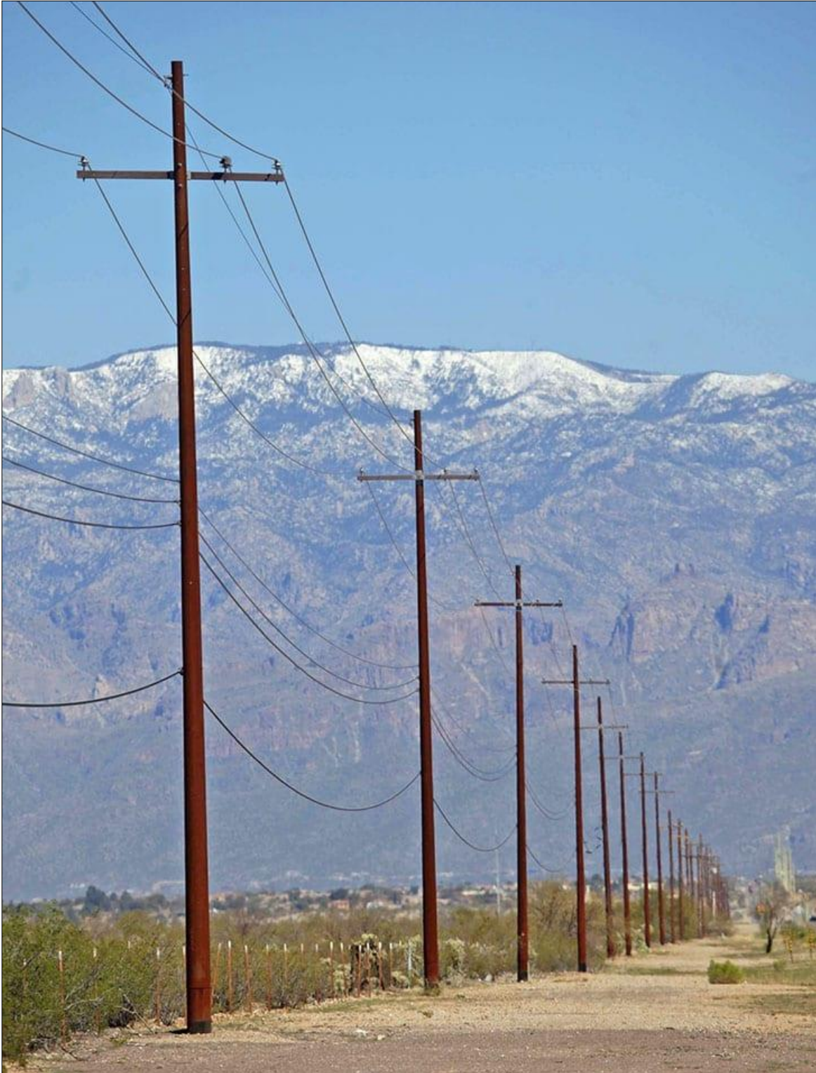
Figure 2: Corten steel transmission poles in a similar monopole configuration as to what would be used for the Project
